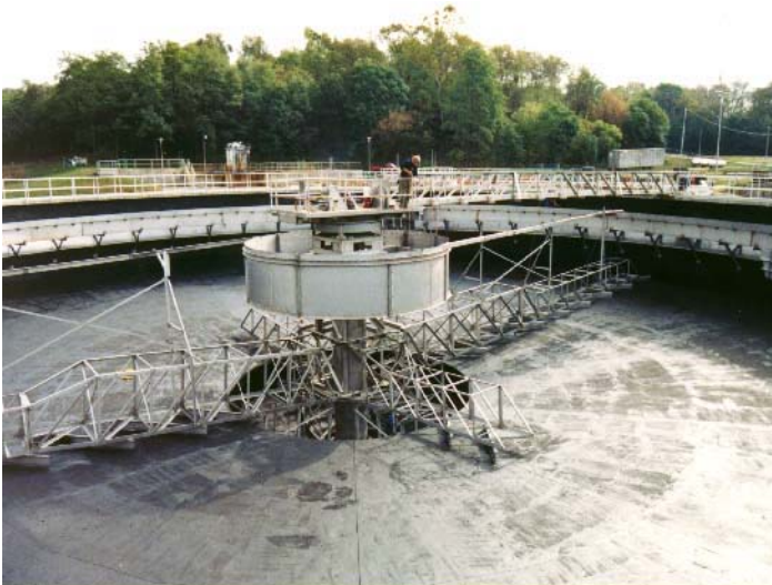
Typical column-supported center feed clarifier.
