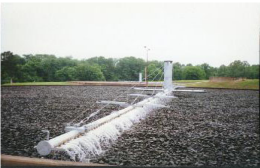
Typical hydraulically-driven rotary distributor.
