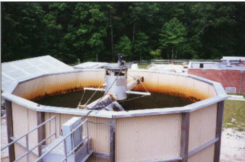
Typical motor-driven rotary distributor.
