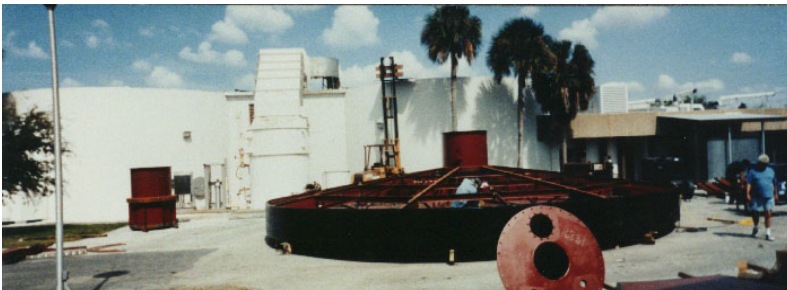
Typical dual deck floating cover.
