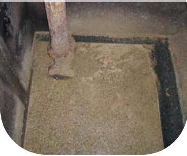
Ft. Collins, Colorado Before: 4" grease
