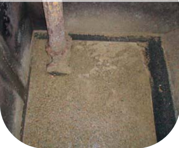
Ft. Collins, Colorado Before: 4" grease
